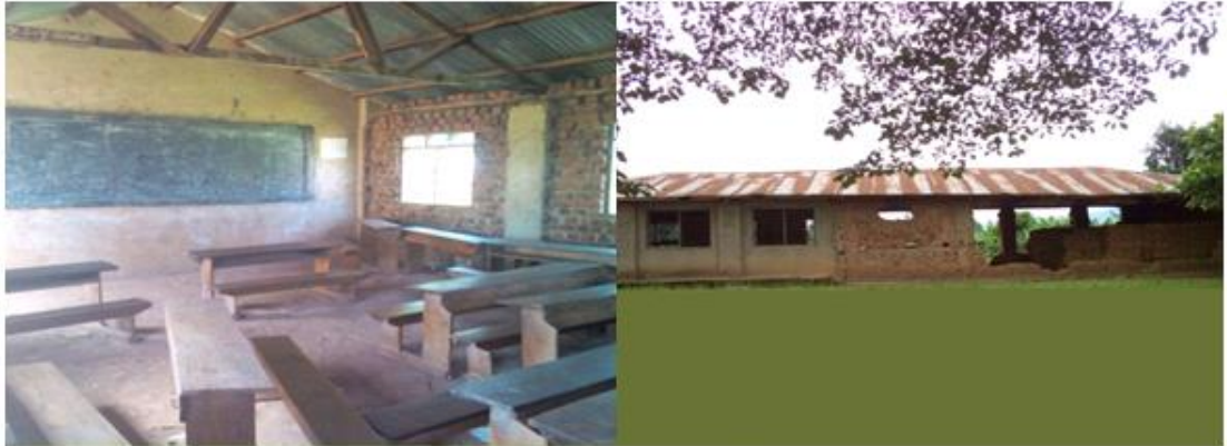
Some of Dilapidated classrooms in some of the visited schools during the survey
