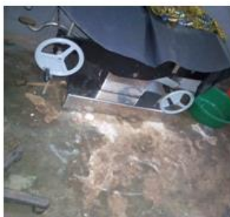
3Dilapidated structures: Delivery Room (Rwimi HCIII)
