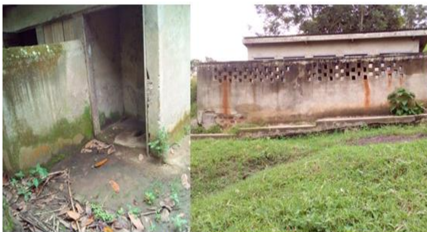
Some of Dilapidated latrines in some of the visited schools during the survey
