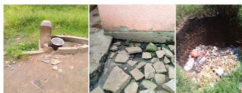
2Dilapidated a bath room at Kibiito HC IV3 Dilapidated water point at Kayenje HCII 1Dilapidated dumping pit at Rwimi HCII
