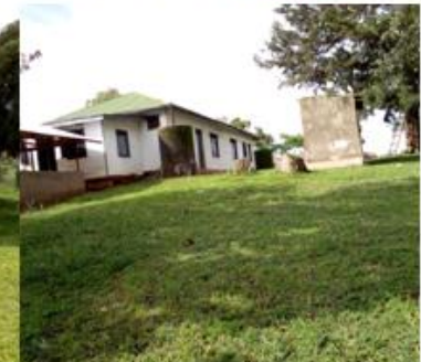
1Dilapidated Structures at Butiiti HCIII
